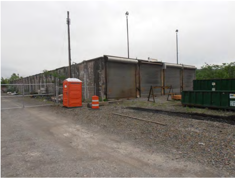
Photograph 10: View of the former Rail Car Thaw Building, located on the western/central portion of the coal storage area on the subject property, looking northeast.
