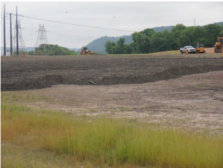
Photograph 6: View of ongoing grading activities associated with the ash impoundment area on the subject property.
