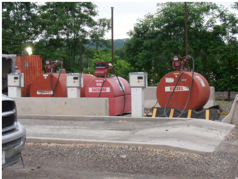
Photograph 21: View of temporary fuel AST's for the Panda Hummel construction, located on the eastern portion for the former coal storage area on the subject property, looking east.
