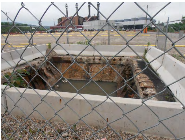
Photograph 18: View of one, of two, coal hopper tunnel openings on the southern portion of the former coal storage area on the subject property. The tunnel openings are secured by fencing.
