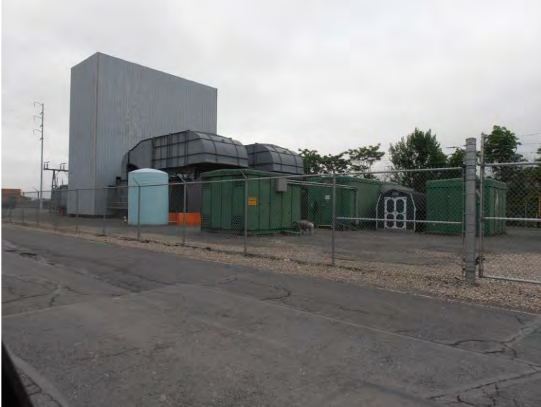
Photograph 12: View of oil fired generators, not on the subject property, south of the Pump House Building.
