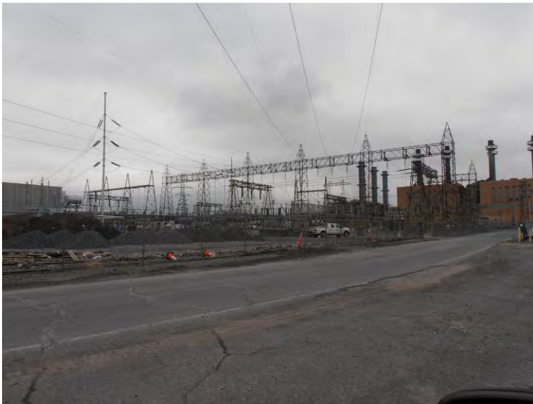
Photograph 13: View of the switchyard, not on the subject property, north of the ash impoundment area. The switchyard is currently undergoing upgrades.
